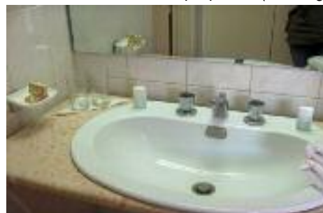
Fig. 1: room taps without mixers
