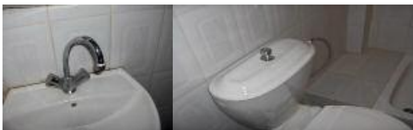
Fig. 1 : taps without mixers and single flushed toilets
